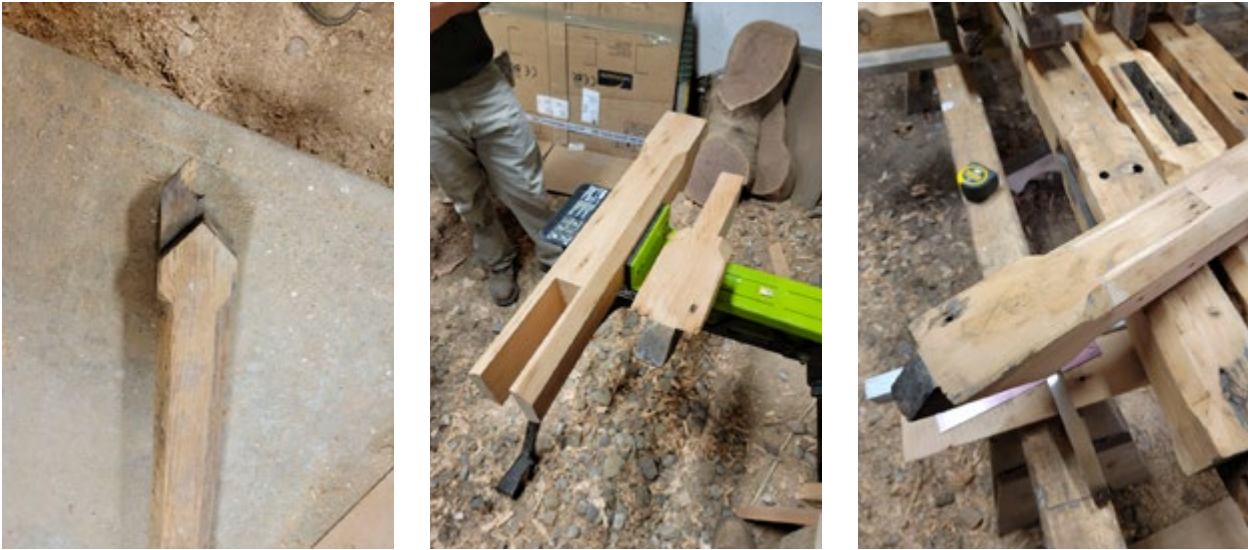
Figures 15, 16 and 17. Brace tenons damaged during installation of the added monitor trusses required blade-and-fork repairs with salvaged ends from damaged braces (Christian & Son, Inc.)
