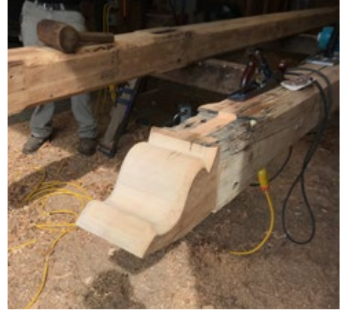
Figures 10 and 11. The decorative ends of timbers removed in the twentieth-century alterations would require replacement, using sections salvaged from other parts of the frame (Christian & Son, Inc.)
