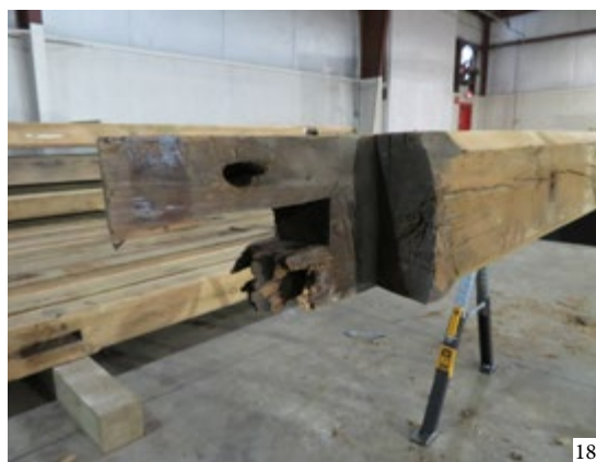
Figures 18 and 19. Damaged scarf joints required repairs that extended back into the solid section of timber (Christian & Son, Inc.)
