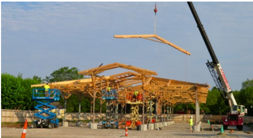
Figure 22. As the historic roof frame sat on top of 15-foot cast-iron and steel columns, installation had to be done with manlifts, extendable forklifts and a crane (Christian & Son, Inc.)
