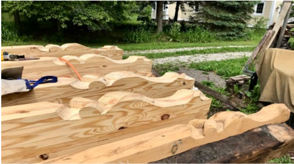
Figure 21. The deeper glulam hip timbers needed matching decorative ends duplicating the original pattern (Christian & Son, Inc.)
