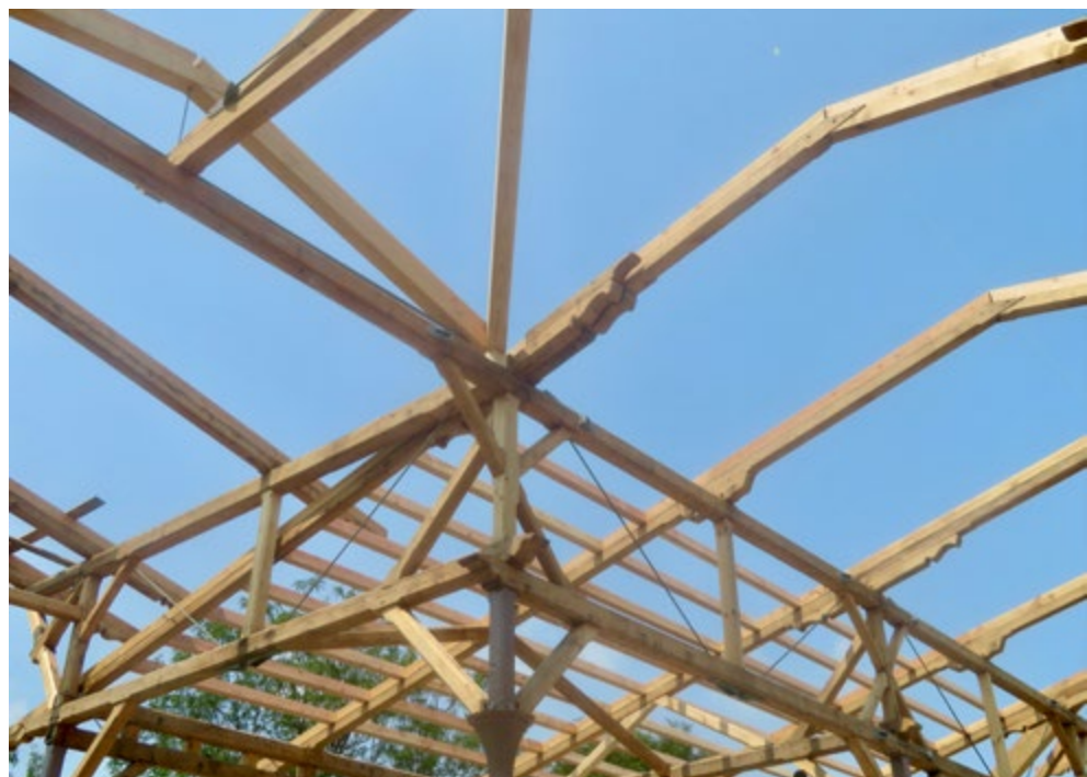
Figure 9. View of the finished frame showing the added compression post/tension rod system installed (Christian & Son, Inc.)
