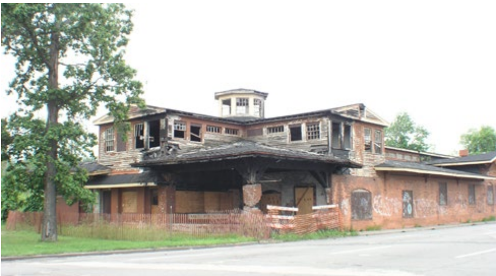
Figure 4. The abandoned Riding Academy building showing evidence of the car crash and ensuing fire as well as general dilapidation in 2003 (Christian & Son, Inc.)
