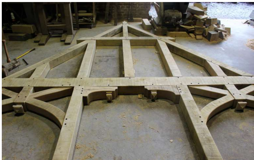
Fabrication of structural elements for the De Wilde–De Scheppe project in Laarne, Belgium
