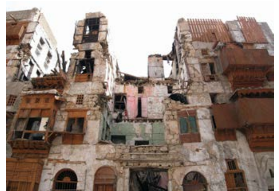
Figure 47: Destroyed building in the old town of Jeddah, which shows the building construction
