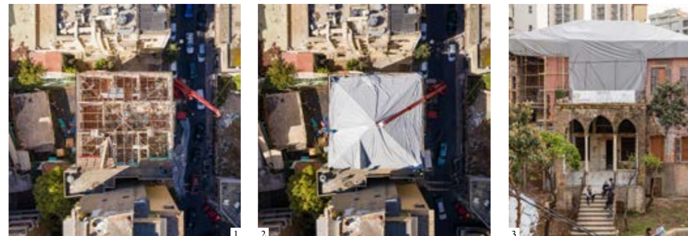
1: Top view of the destroyed pitched roof 2: Covering of the pitched roof with temporary tarpaulin 3: Sheltered roof and triple arched bay (1, 2: Live Love Beirut (LLB) 3: Dia Mrad)
