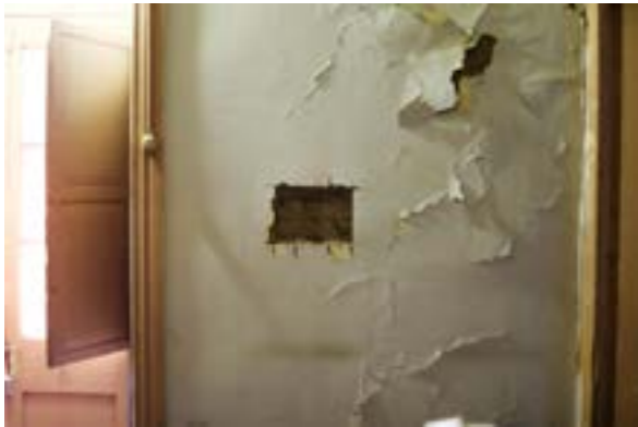
Figure 19: Detachment of synthetic paint layers due to damp retained in the wall. Pathology found in a wall at the Corazón de Maria Convent in Ovalle in 2019
