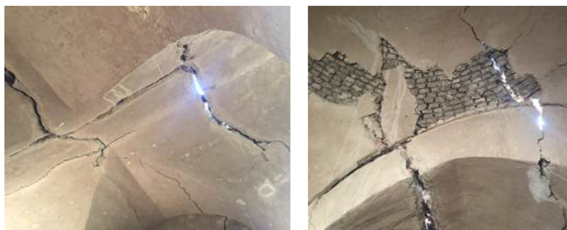
Figure 8: Cracked ceilings | Techos agrietados | Tetos com fissuras
