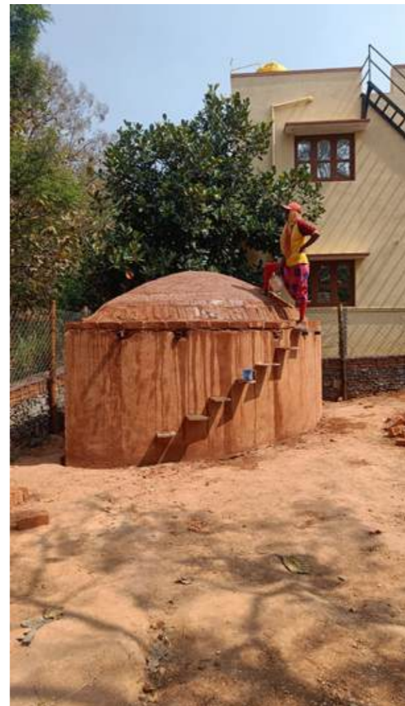
Figure 4: Thappi plastering on a brick and lime mortar water tank (Bagalur, India, 2023)
