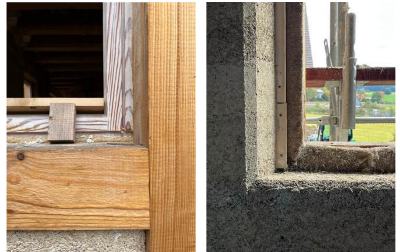
Window detail from outside and from inside | Detalle de la ventana desde el exterior y el interior | Pormenor da janela vista do exterior e do interior
